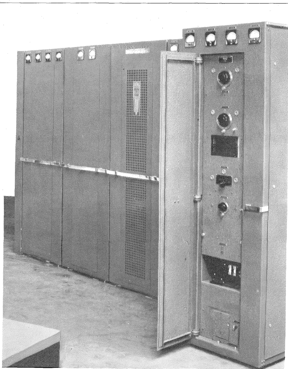
Fig. 2—Five Kilowatt Multi-Unit Equipment. R. F. Door Open.
